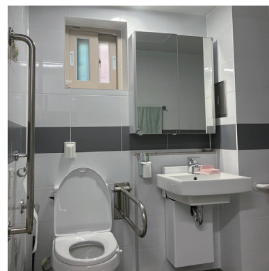
Bathroom for older persons: automatic height-adjustable washbasin and ceiling heater
