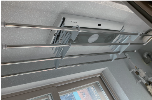
Automatic height-adjustable drying rack in patio
